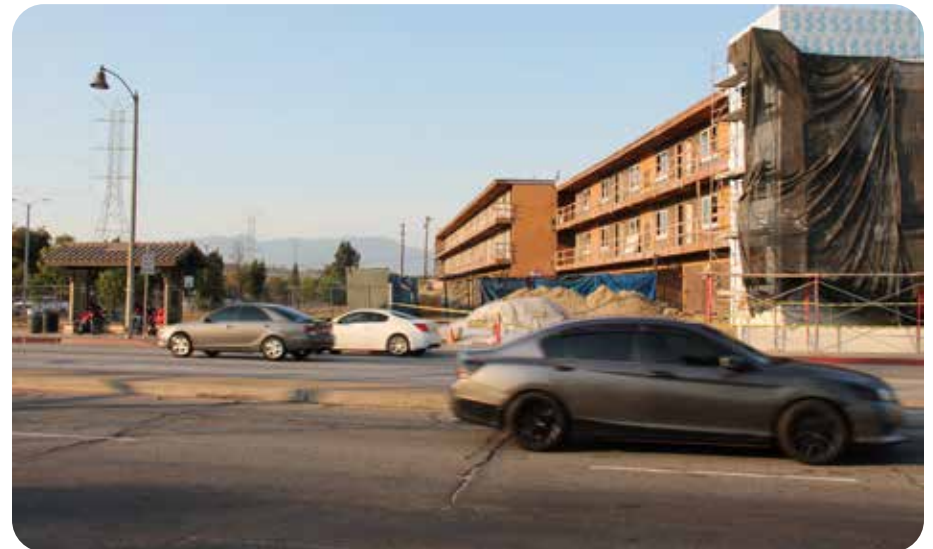
Current renovation of multi-family residential building at the corner of Whittier Boulevard and Paramount Boulevard.
