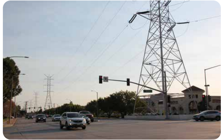
Major high-voltage transmission lines head north-south along the west side of Paramount Blvd through the City and Specific Plan Area.
