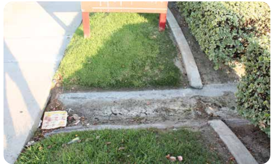
Drainage channel from parking lot through landscape area directed under sidewalk to Whittier Boulevard.
