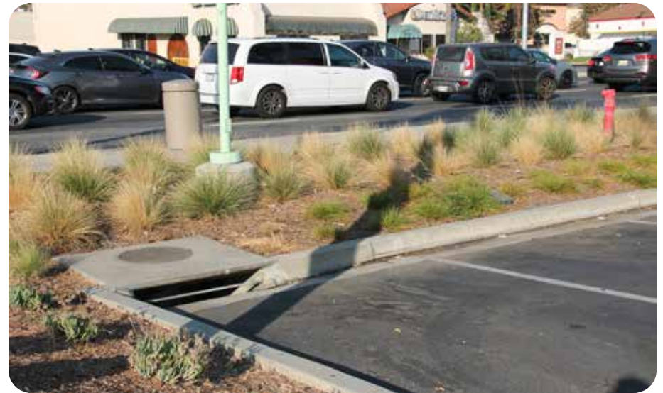
Stormwater runoff directed to sewer system instead of adjacent planting area.
